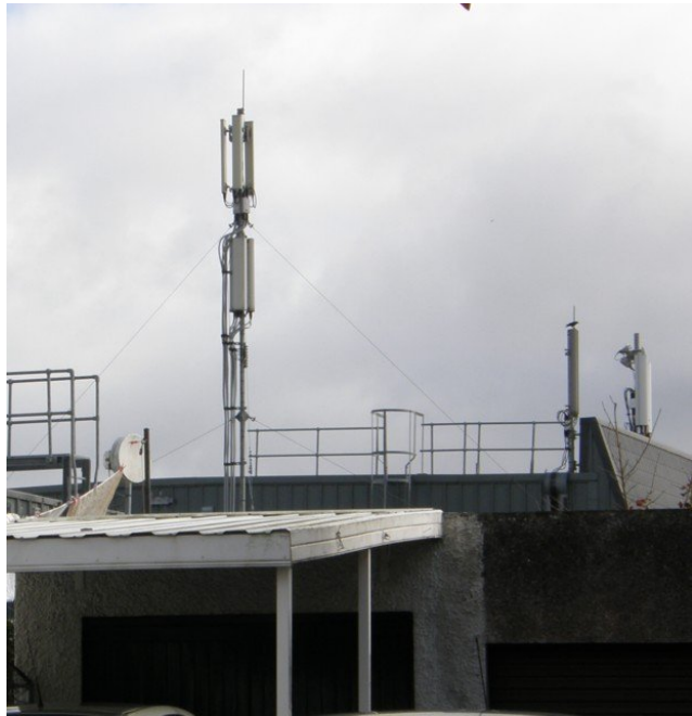
Transmitter Site Photo
